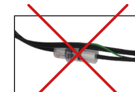
Water trap NOT OK
